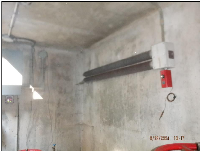
Photo 4 – Valve Chamber Interior
