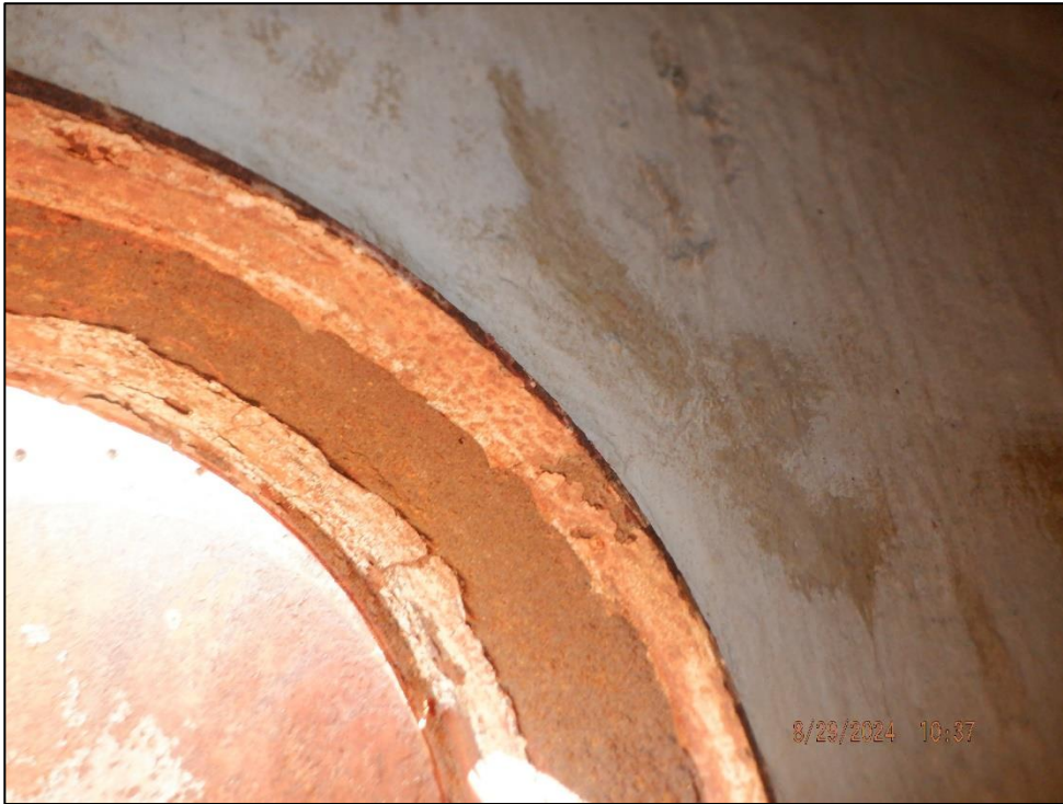
Photo 9 – Corrosion on Steel Access Door
