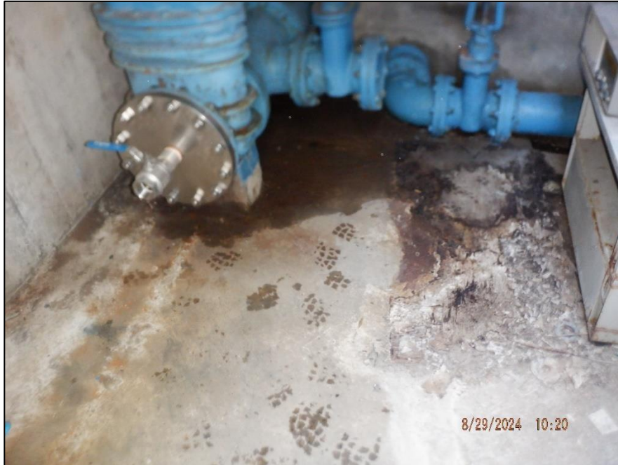
Photo 6 – Moisture Accumulation in Valve Chamber
