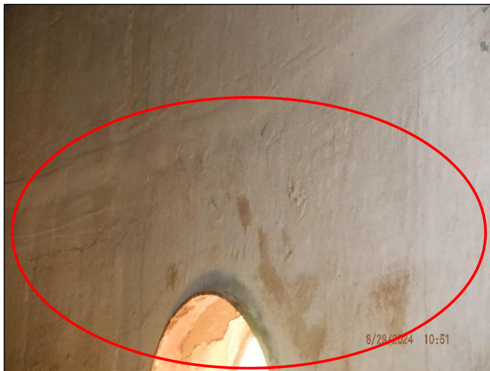
Photo 10 – Patch Around Access Door
