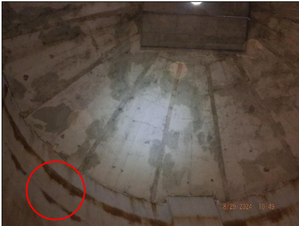
Photo 8 – Corrosion Staining at Compression Ring
