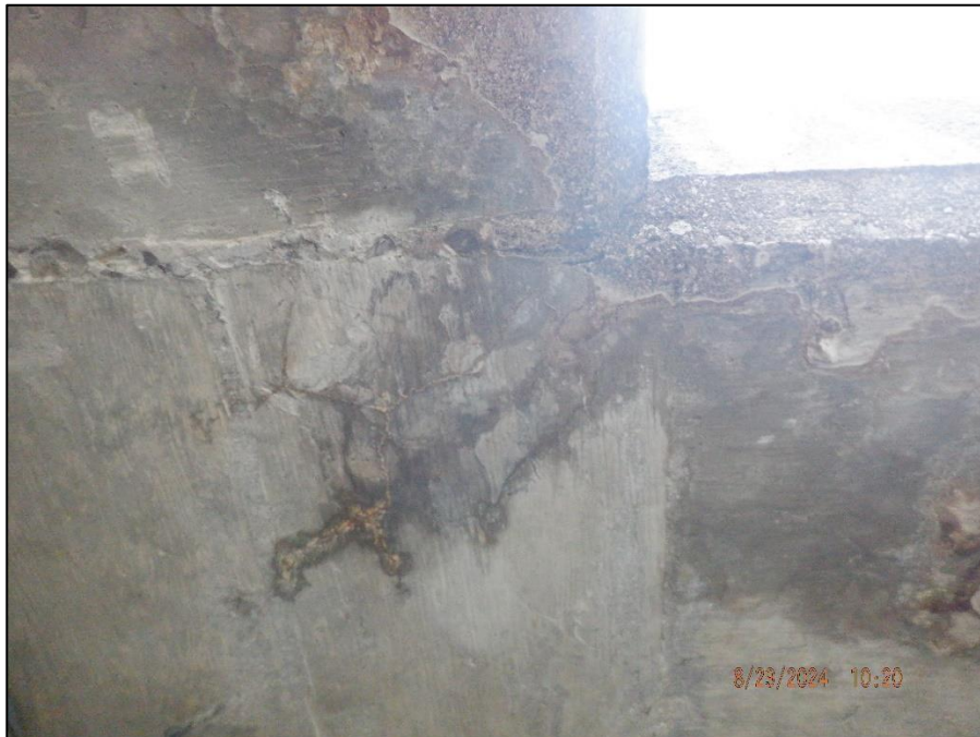
Photo 7 – Cracking with Efflorescence on Valve Chamber Soffit
