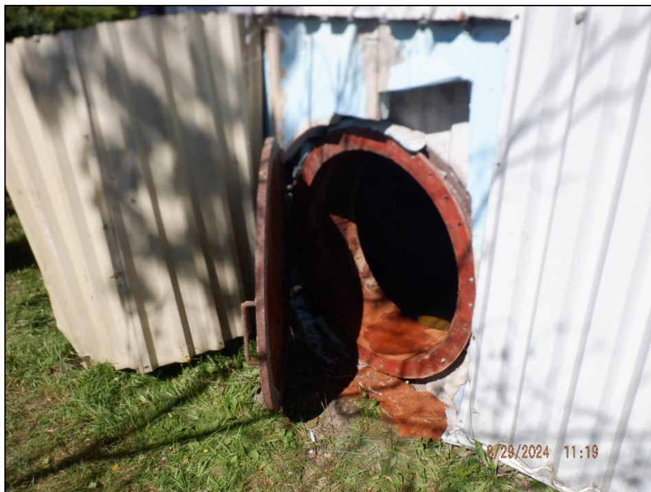
Photo 3 – Access Door Behind Siding
